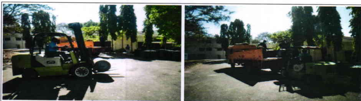
PCB dechlorinated oil is loading into the TNEB vehicle
