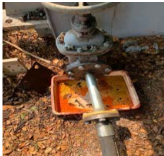
Figure 33: Oil drain line and suction line connection
