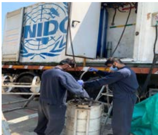
Figure 36: Loading of sodium dispersion drum
