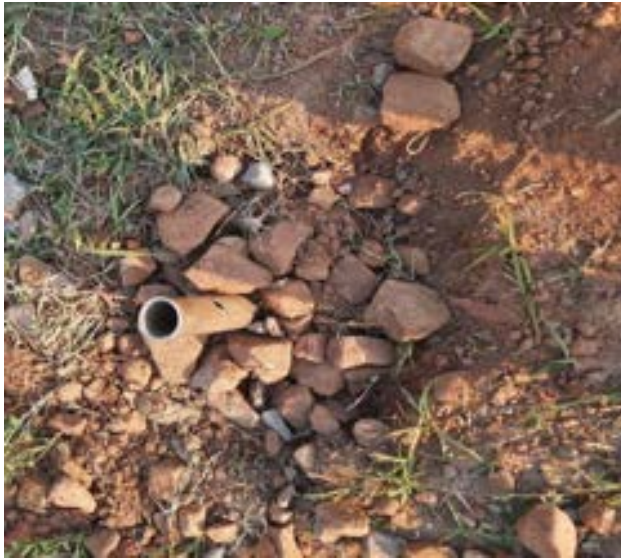
Figure 7: Earthing pole Installed.
