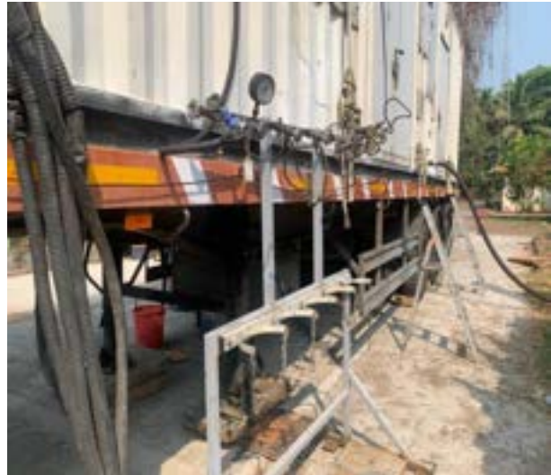
Figure 19: Nitrogen manifold connected to PCB unit
