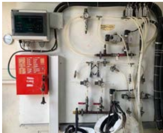
Figure 23: Checking the nitrogen gas line control
