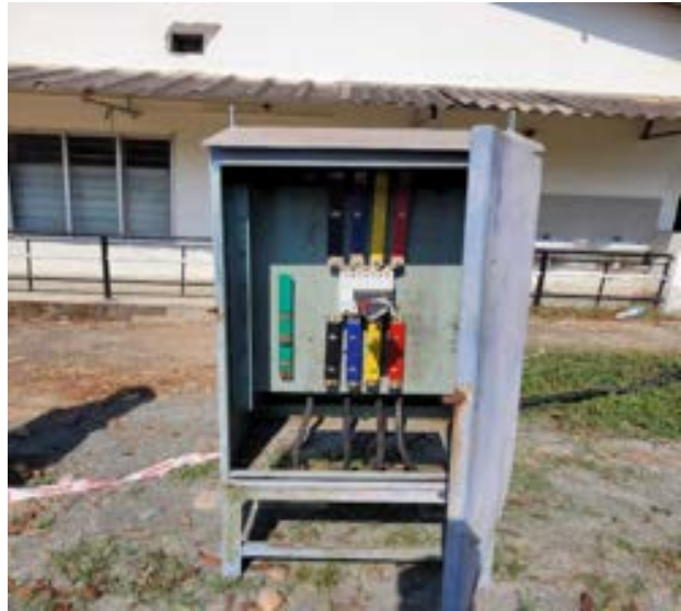
Figure 8: Power circuit breaker box.
