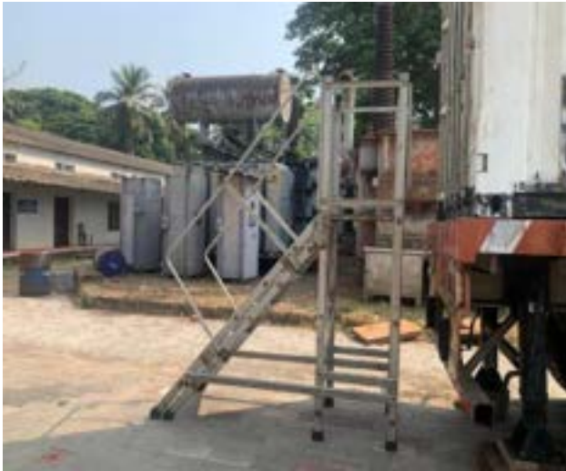
Figure 18: Ladders fixed to the PCB unit
