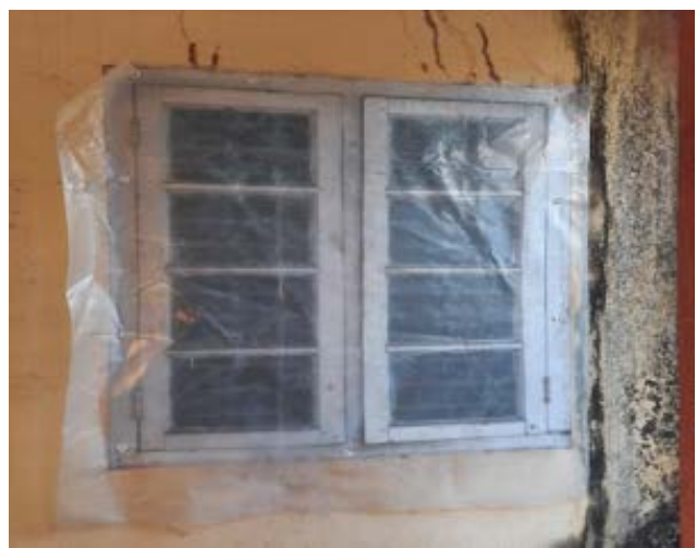
Figure 10: Window of the room closed with plastic sheet to avoid rainwater.
