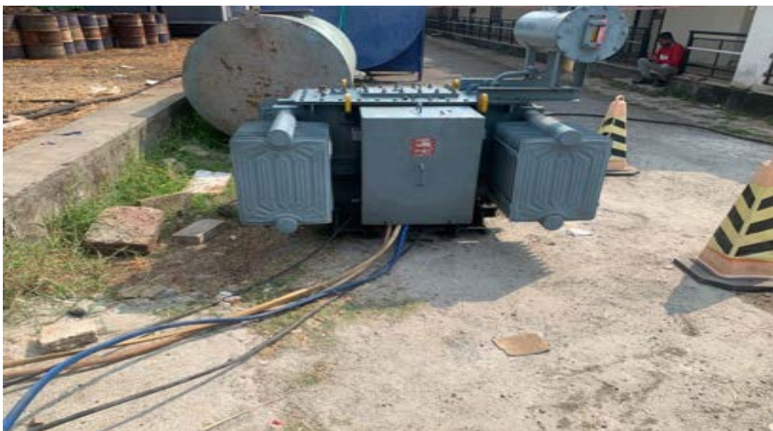
Figure 20: The step down transformer connected to PCB unit.
