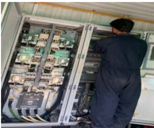
Figure 22: Checking the Electrical connections for main control panel
