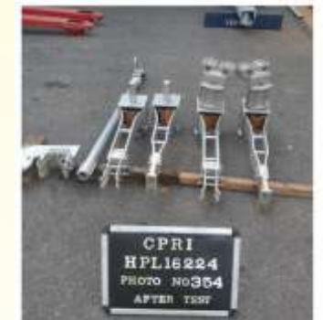
123 kV Center break disconnect of M/s. Costar switchgear, Chennai was tested for short time withstand current test of 31.5 kA for 3 sec.
