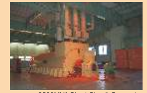
2500MVA Short Circuit Generator
