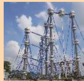
HVDC Generator at UHVRL, Hyderabad
