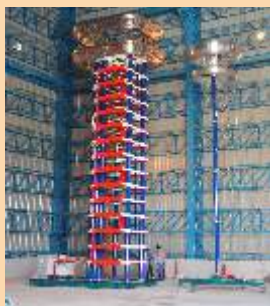
2400kV, 240kJ Impulse Voltage Generator
