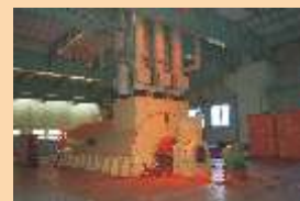
2500MVA Short Circuit Generator
