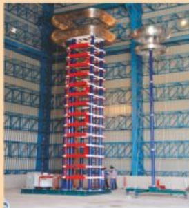
2400kV, 240kJ Impulse Voltage Generator
