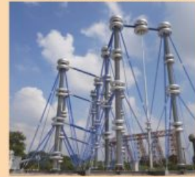
HVDC Generator at UHVRL, Hyderabad
