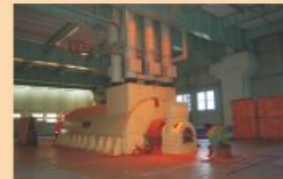
2500MVA Short Circuit Generator
