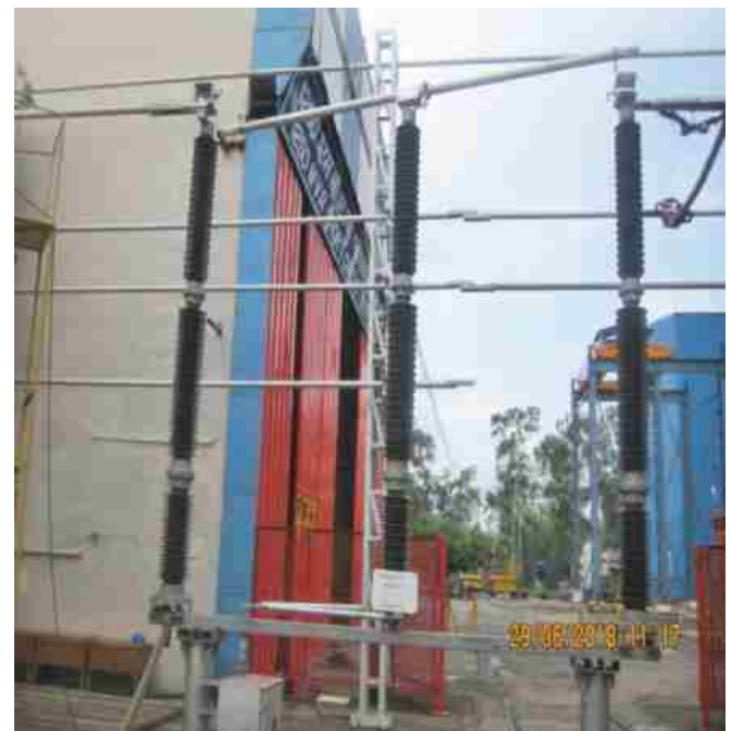
Short time withstand current and Peak withstand current test at 63kArms for one second with initial peak of 158kA as per Clause 6.6 of IEC: 62271-102, 2001 on 420 kV , 3150A Horizontal Double Break Disconnecter carried out at STDS-CPRI, Bhopal for GR Power Switchgear Limited, Hyderabad
