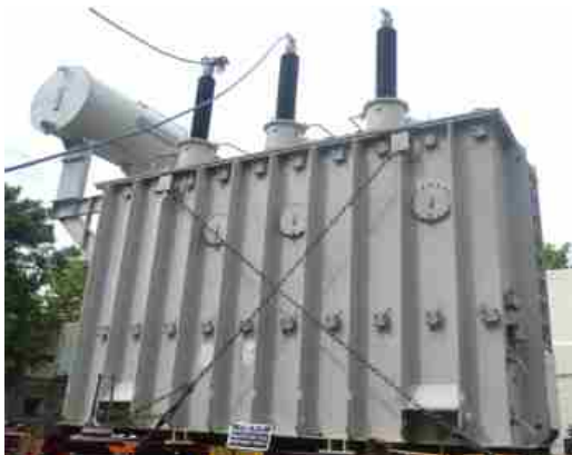
Ability to withstand the dynamic effects of short circuit test on 80/120MVA,132/33kV, Three Phase Transformer carried out at High Power Laboratory, CPRI, Bangalore
