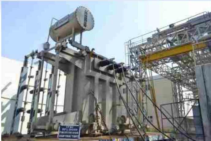
Ability to withstand the Dynamic Effects of Short Circuit test on 5 MVA, 33 kV/0.360-0.360 kV, Three Phase Transformer for M/s. Shilchar Technologies Limited, Vadodara
