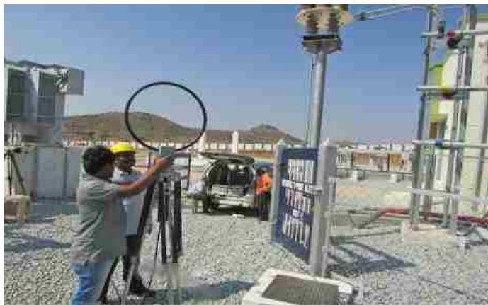
Measurement of Radio Interference Voltage (RIV) around 100 MVAR, STATCOM unit, for 400/220kV, PGCIL substation, NP Kunta, Anathapur, AP
