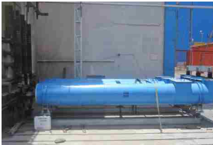
Short time withstand current test at 90kArms for one second with initial peak of 230kA as per IS: 8084 on 11 kV , 4000A, 90kArms Busduct for M/s. BHEL, Rudrapur carried out at STDS-CPRI, Bhopal
