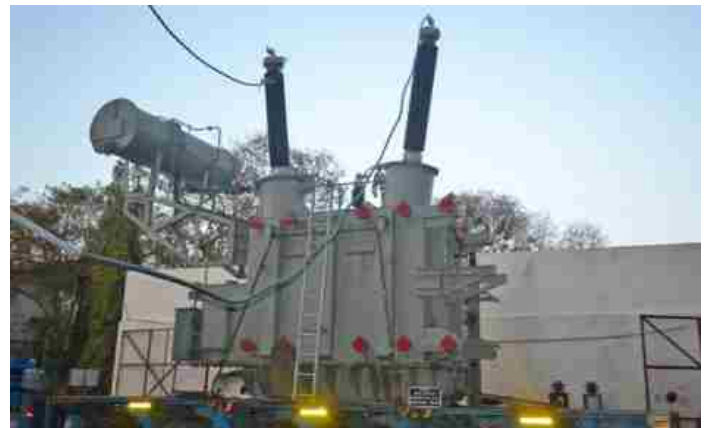
Ability to withstand the dynamic effects of short circuit test conducted on 30.24 MVA, 220/27 kV single phase traction transformer for M/s. Transformers & Rectifiers Ltd., Ahmedabad at High Power Laboratory, CPRI, Bangalore
