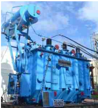
Ability to withstand the dynamic effects of short circuit tests on 35 MVA, 23.5/11.5 kV Three phase oil filled power transformer carried out at High Power Laboratory, CPRI, Bangalore
