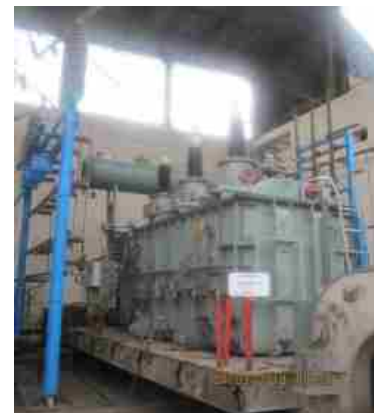
Short Circuit Dynamic withstand tests as per Clause 4.2 of IS 2026 (Part-5), 2011 conducted on 25/31.5MVA, 66/11kV Power Transformer for M/s. Technical Associate Ltd., Sitarganj at STDS-CPRI, Bhopal
