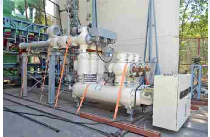
Short-time withstand current test on 245 kV, 3150 A, 50 kA GIS for M/s. Siemens Ltd., Aurangabad, Maharashtra
