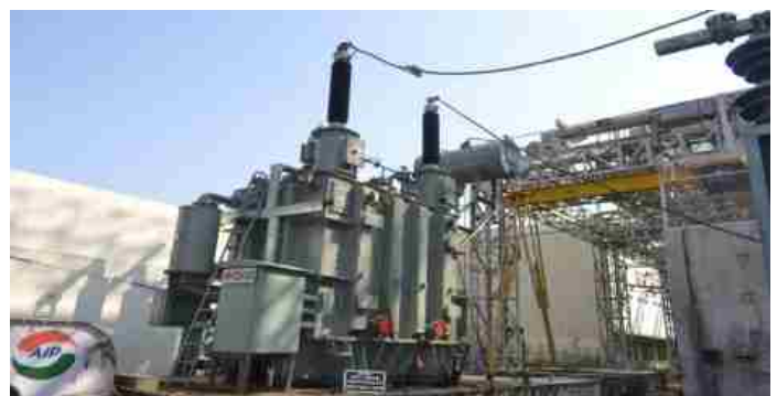
Ability to withstand the dynamic effects of Short circuit test on 21.6 MVA, 132 kV/27 kV Single Phase Transformer for M/s. Vishvas Power Engineering Services Pvt. Ltd., Nagpur
