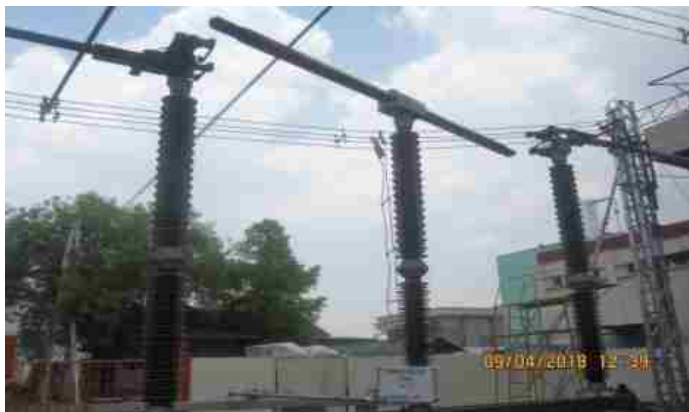
Short time withstand current and Peak withstand current test at 63kArms for three second with initial peak of 163.8kA as per Clause 6.6 of IEC: 62271-102, 2001 on 300kV, 4000A Horizontal Double Break Disconnector for M/s. ABB India Ltd., Vadodara carried out at STDS-CPRI, Bhopal
