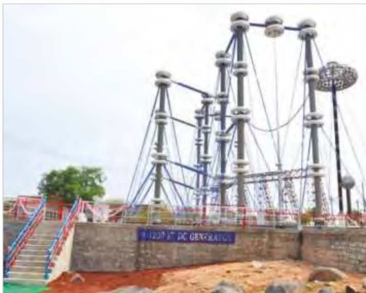
A View of ± 1200 kV DC Test System
