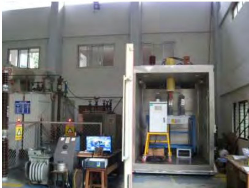
A view of the tested 38 kV, 1200A Autorecloser
