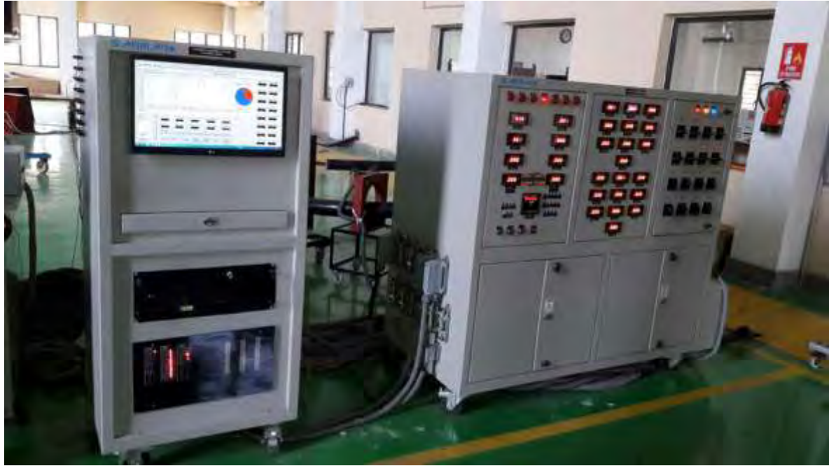
Control panel for current loading system
