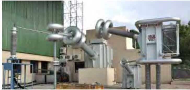
600kV, 4200 KVA Outdoor Transformer
